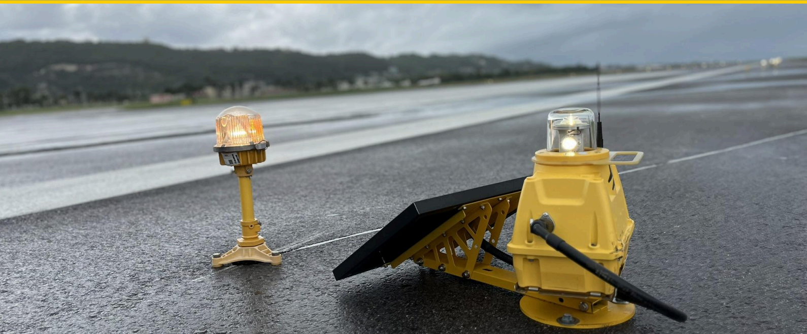
S4GA solar-powered runway edge light (right) installed as a backup for a conventional light (left)
