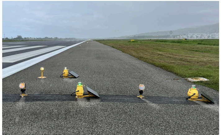
S4GA solar backup airfield lighting system installed at Sangster International Airport, Jamaica
